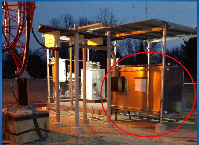
WROK-AM, Custom Isocoil Installation
