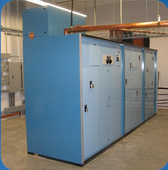
Floor mounted single or multibay phasor cabinet with front and rear access
