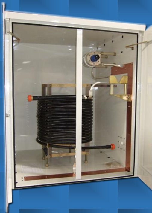
Kintronic Custom FM Isocoil for FM antenna feed on AM tower
