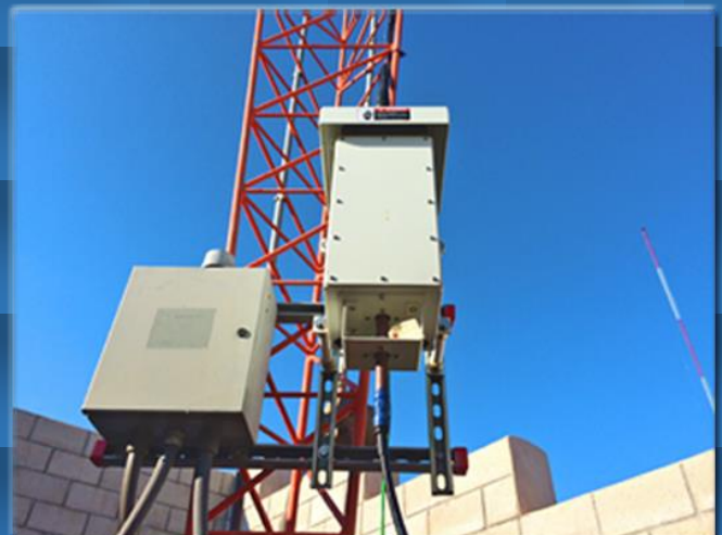
FMC-1.5 Isocoupler for FM antenna feed on AM tower
