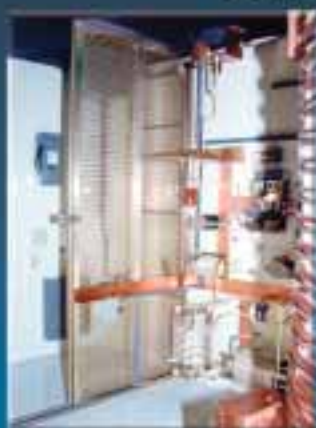
Installed in KTL Prefabricated Building
