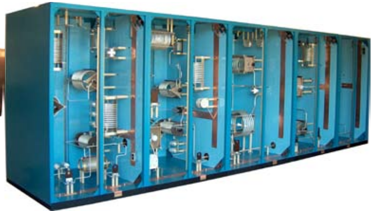
PHASOR CABINET REAR VIEW WITH DOORS REMOVED
