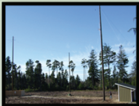
Overview of KinStar Antenna Showing Center Support w/Fence on Left & XMTR on Right
