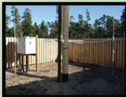
Antenna Tuning Unit Installed at Base of Center Support
